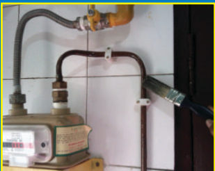
PNG PIPE LINE
